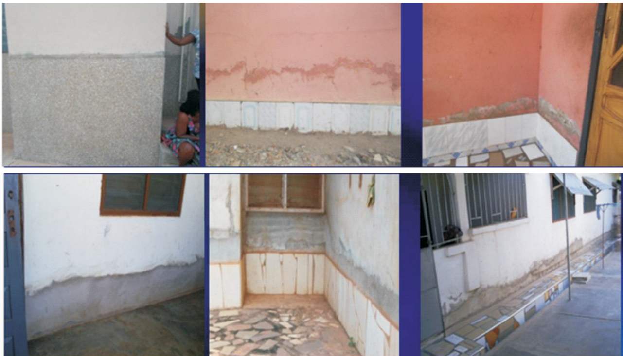
FIGURE 6.0: Ways in which rising damp is controlled in Ghana
